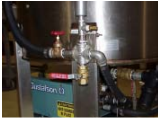
Treatment supply tank valve and bypass system
