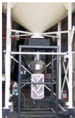
Weighing Bin & Frame
